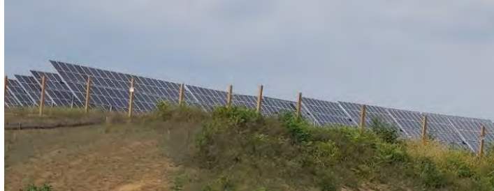
Chambersburg Solar Center – Photovoltaic Panels
