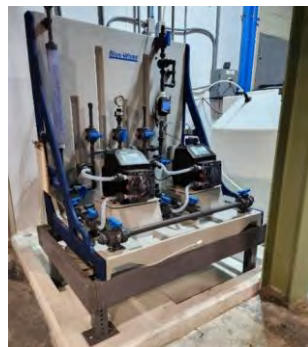
New Chemical Feed Equipment Installed in 2023
