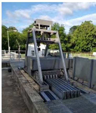
Aging Equipment – UV Disinfection
