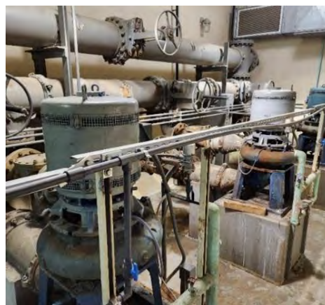
Aging Equipment – Old Headworks
