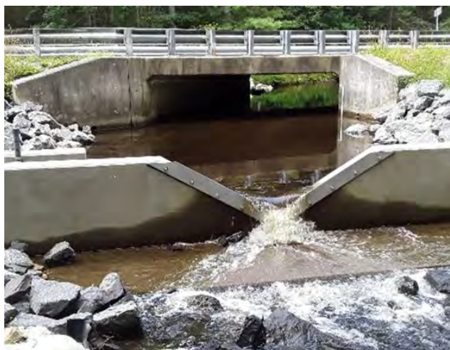
Conococheague Weir in Operation
