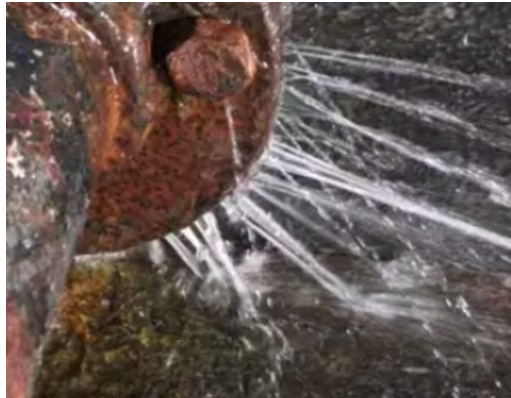
Water leaking from a flange seal
