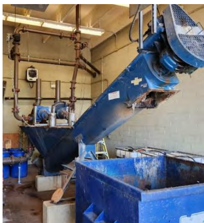
Aging Equipment – Grit Removal
